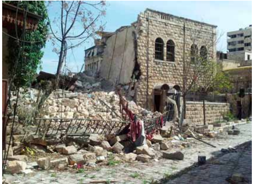
The damaged building of the Presbyterian church of Aleppo. Photo: NESSL
